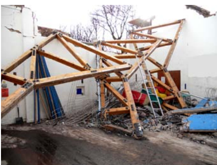
School roof collapse
