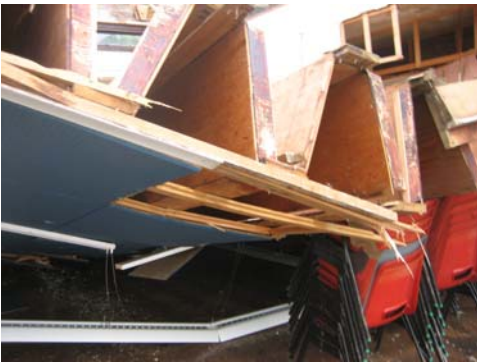
Collapse of Timber Roof
